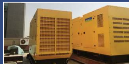
Allied Bank 2x500kVA
